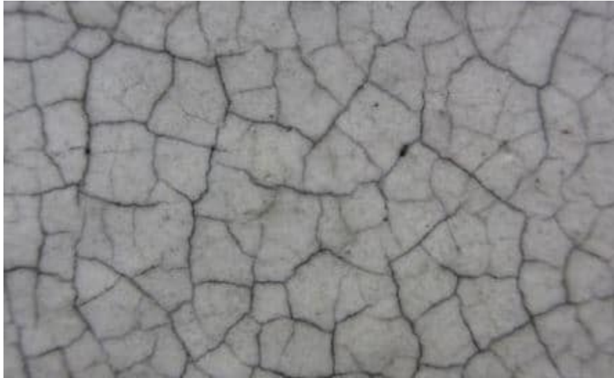
Fig -Crazing or Pattern Cracking
